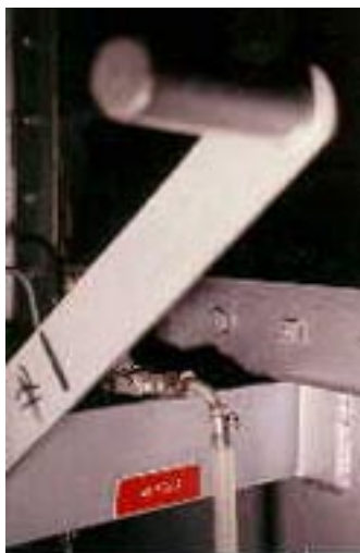
Ammonia injection system
